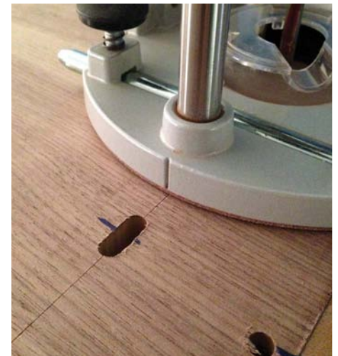
Rout slots in the carcass top so the bolts can move freely if so required
